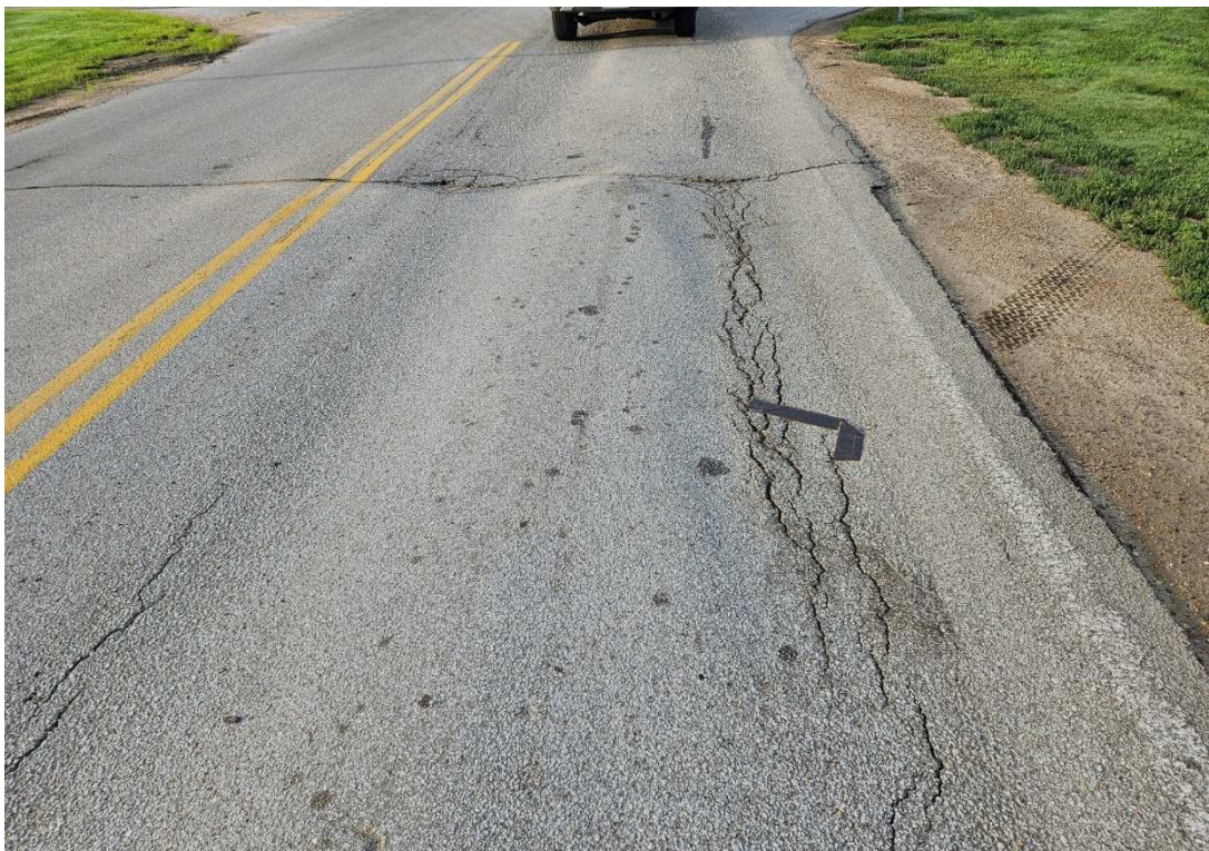
FIGURE 5.2: 2 ND ST, RUTTING & LONGITUDINAL CRACKING IN WHEEL PATH AT HIGHWAY 92
