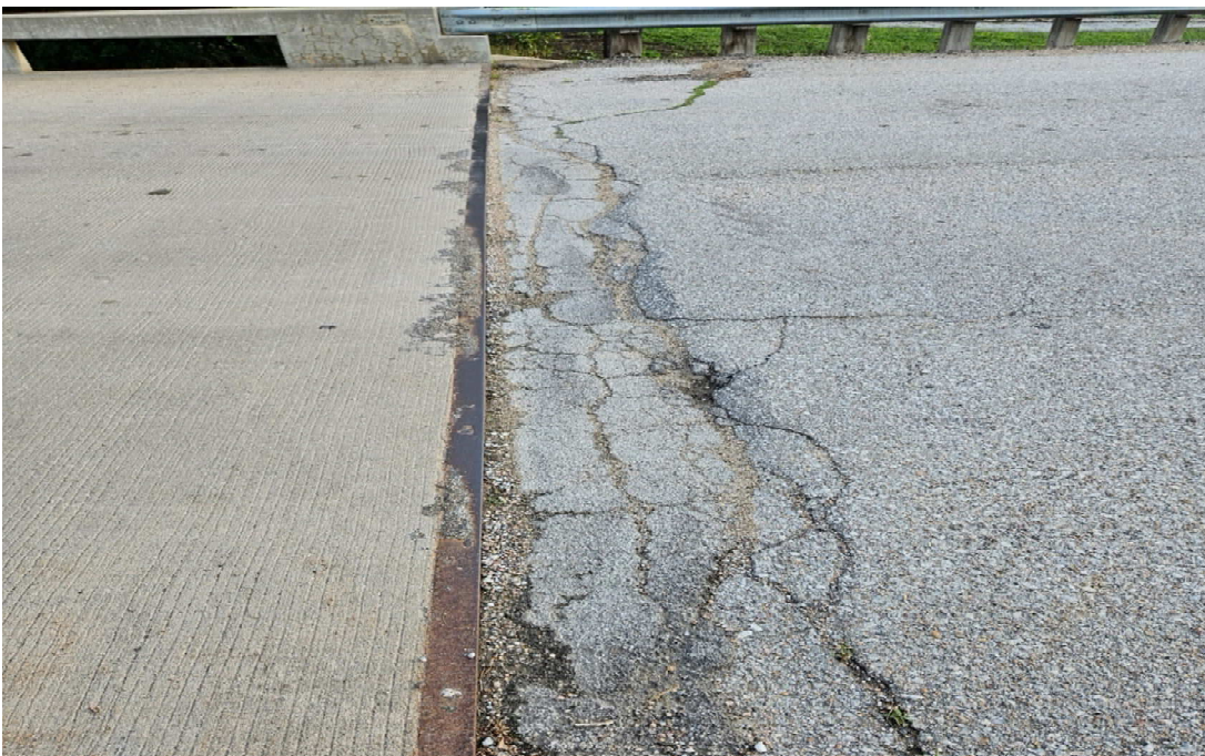
FIGURE 5.12: VINE ST, CRACKING & SETTLEMENT AT THE EAST DECK JOINT OF THE BRIDGE OVER UPPER CLEAR CREEK
