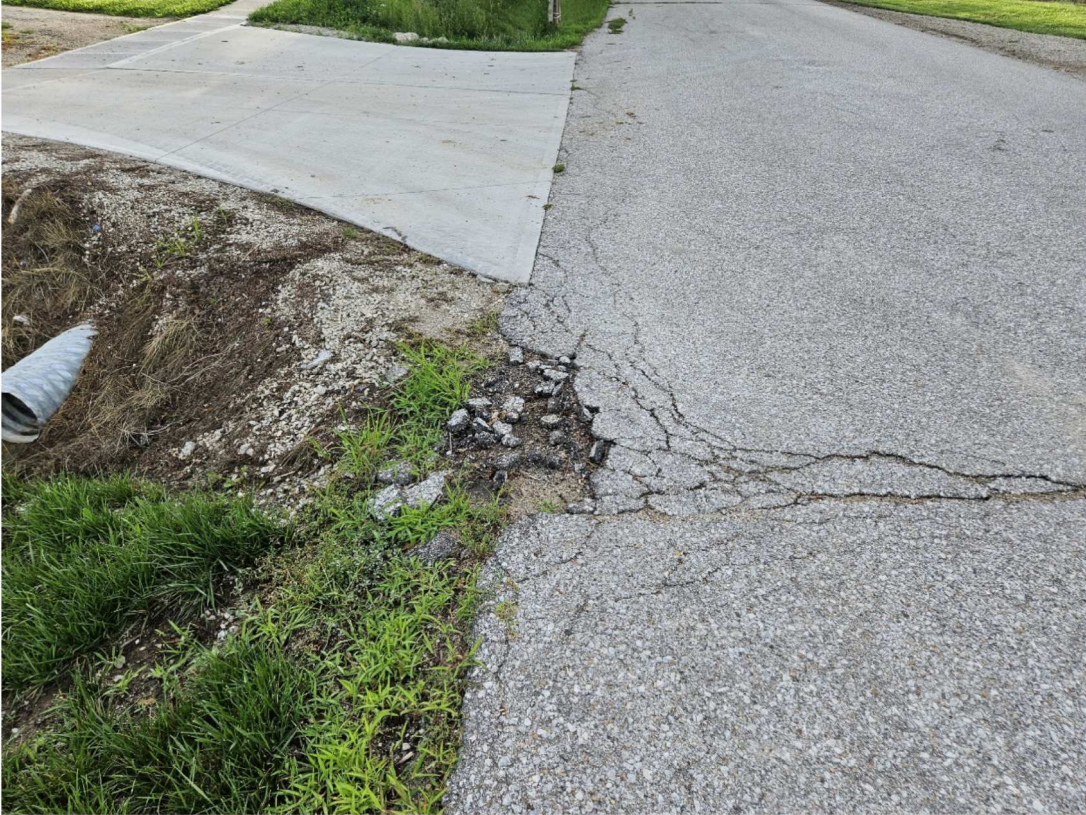
FIGURE 5.15: VINE ST, EDGE FAILURE
