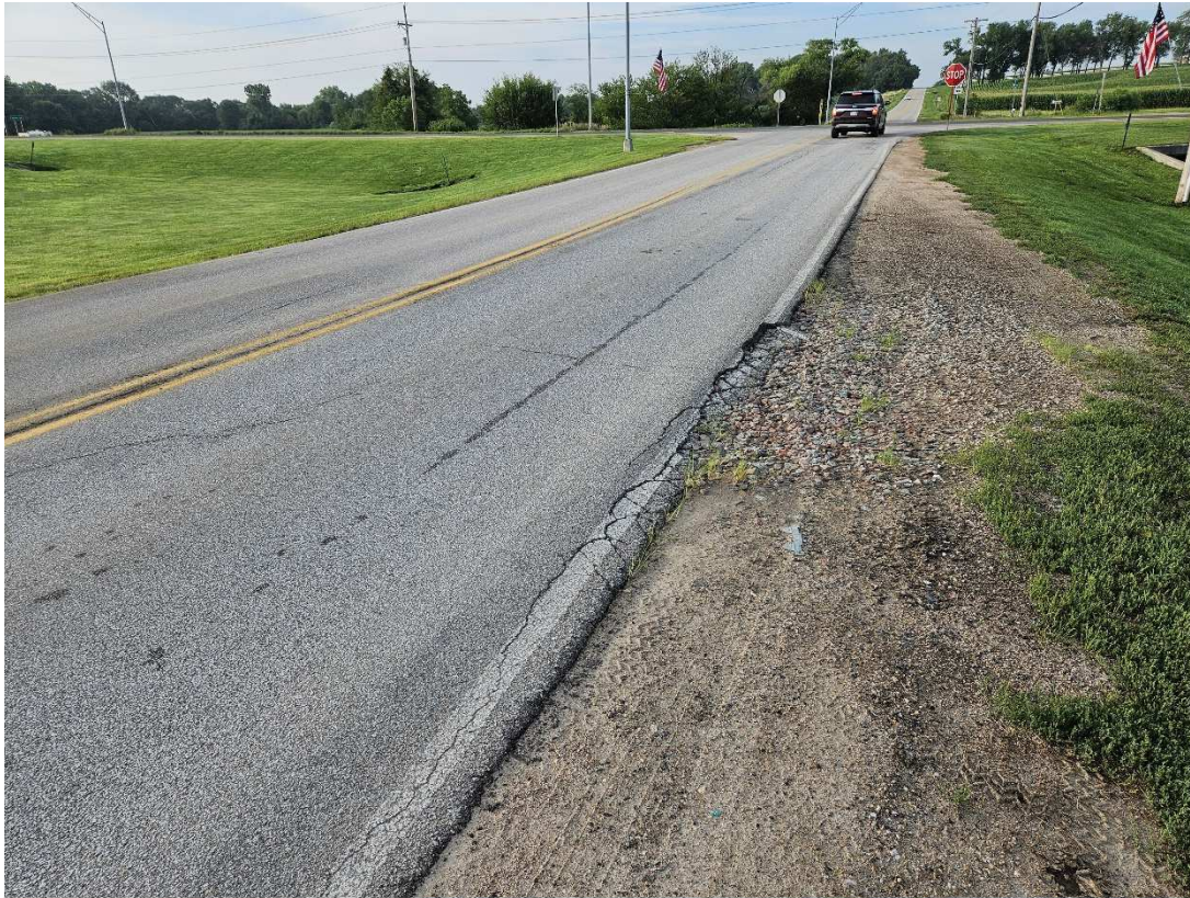
FIGURE 15.3: 2 ND ST, EDGE FAILURE
