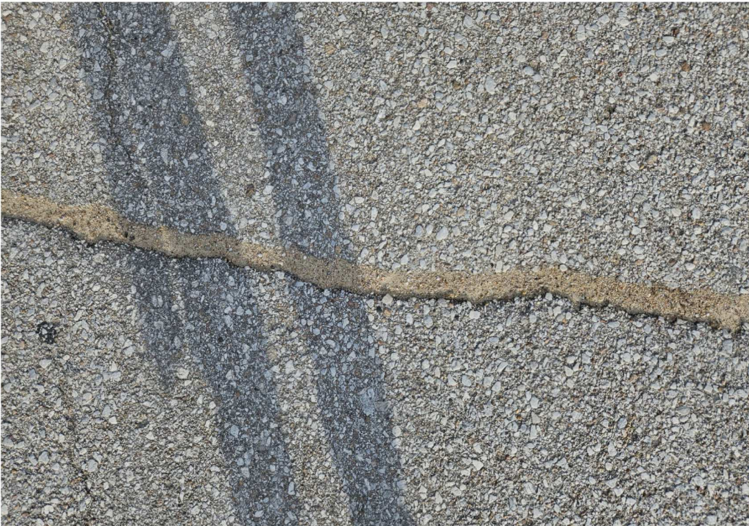
FIGURE 5.16: VINE ST, WIDE TRANSVERSE CRACKING
