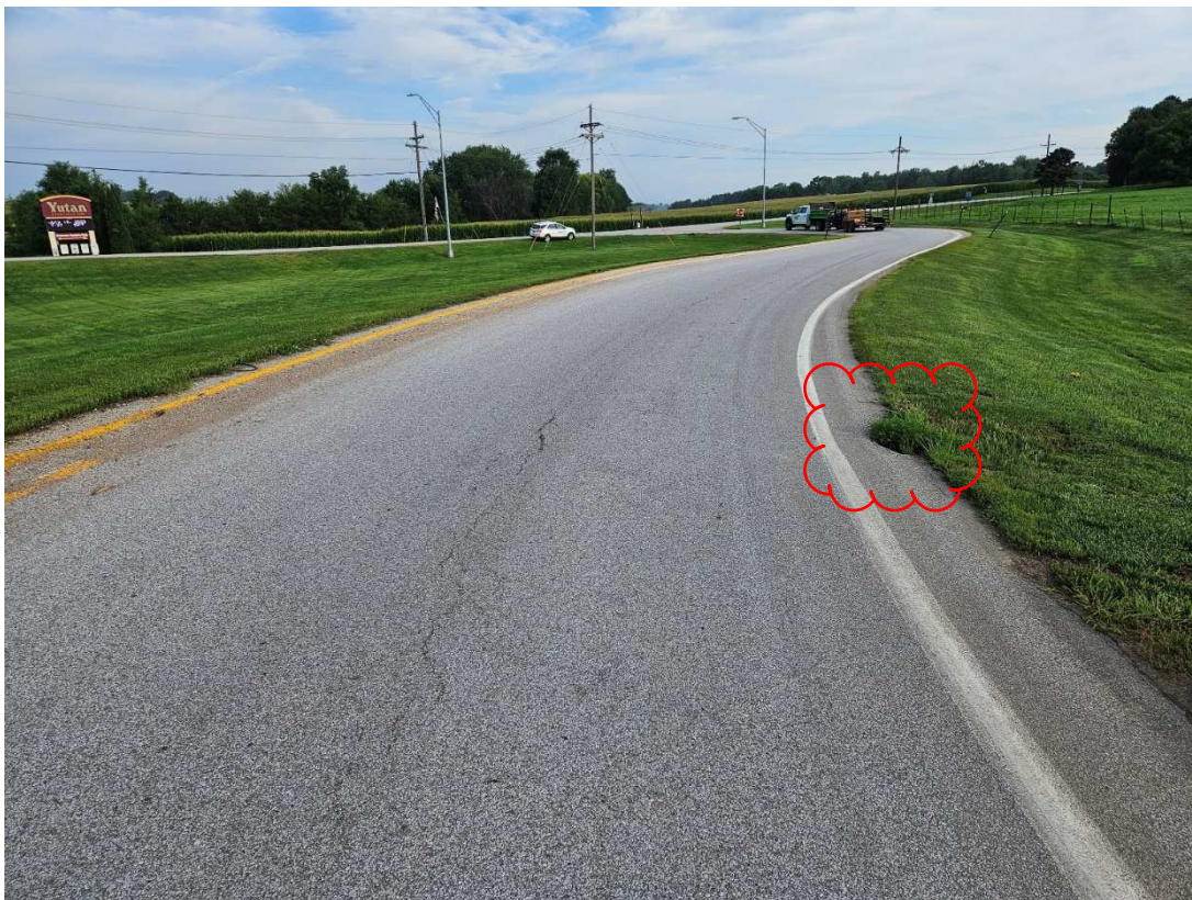
FIGURE 5.8: 092RA, SINKHOLE ON EAST SHOULDER
