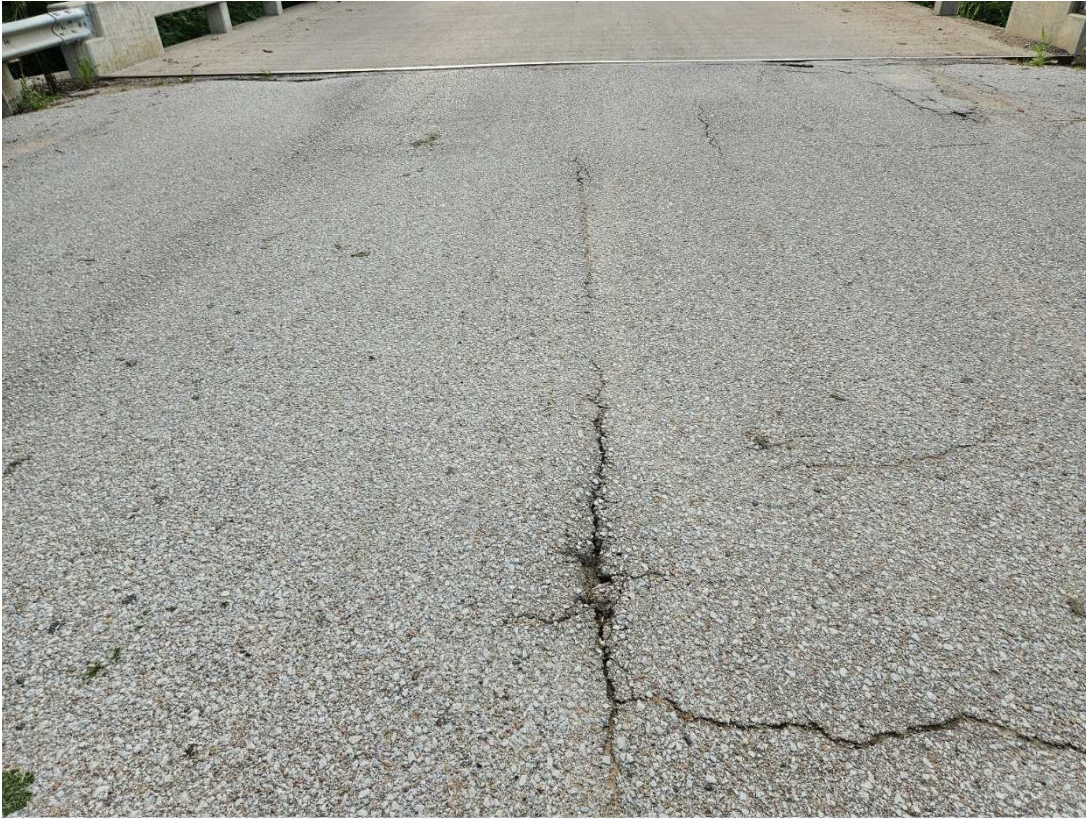
FIGURE 5.11: VINE ST, LONGITUDINAL CRACKING
