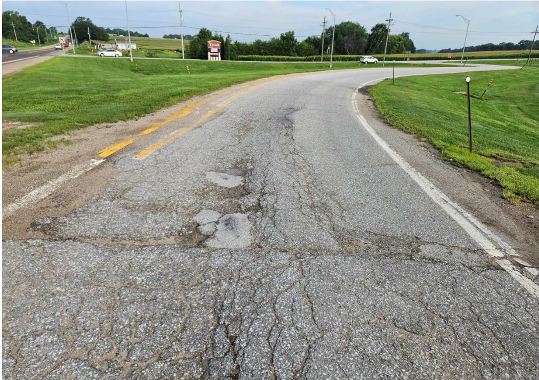
FIGURE 5.7: 092RA, PAVEMENT DISTRESSES NEAR HIGHWAY 92
